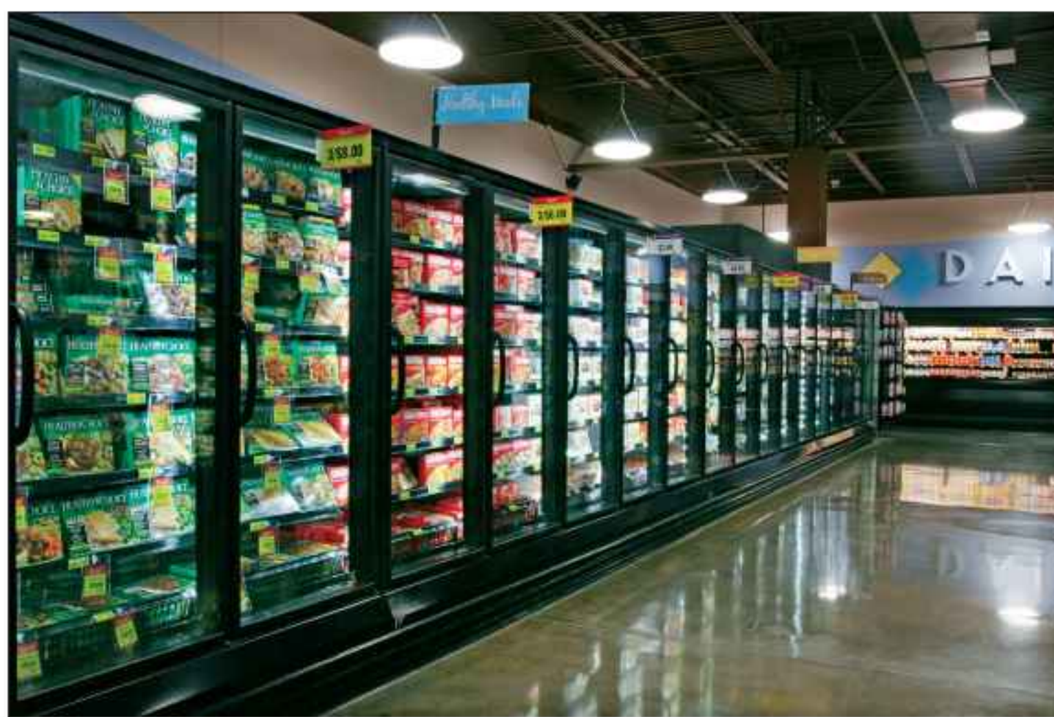
Refrigerated display case doors in United Supermarkets' stores.
