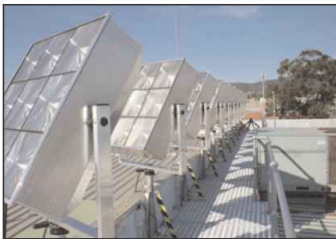
SunCubes in a roof-mounted installation.
