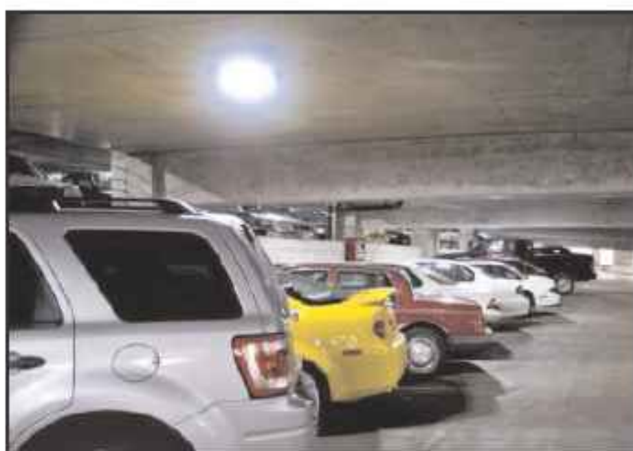
Parking deck in six-storey garage retrofitted with LED lighting.
