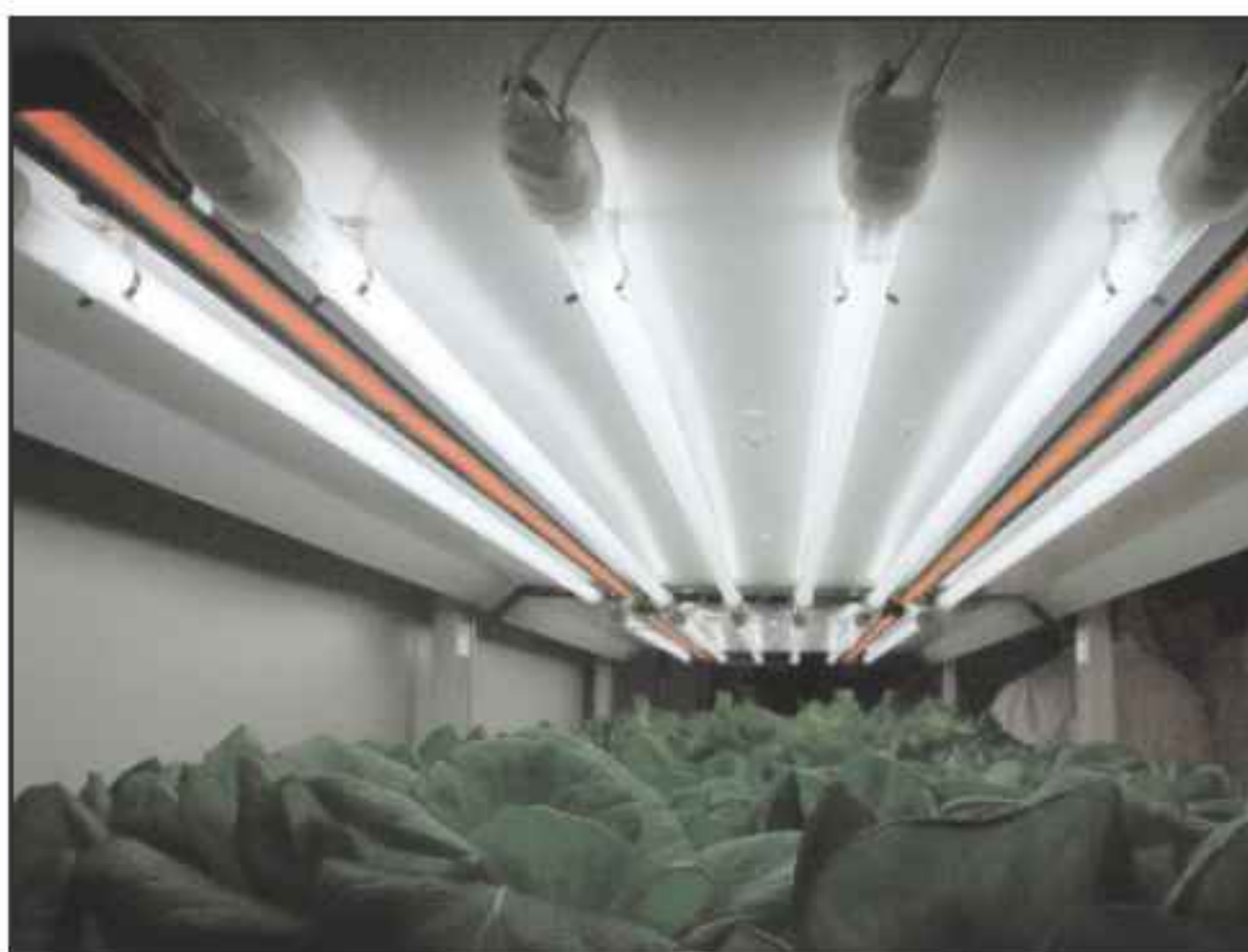
Lamps using red LED chips (which are best suited for plant growth), alongside fluorescent lamps.
