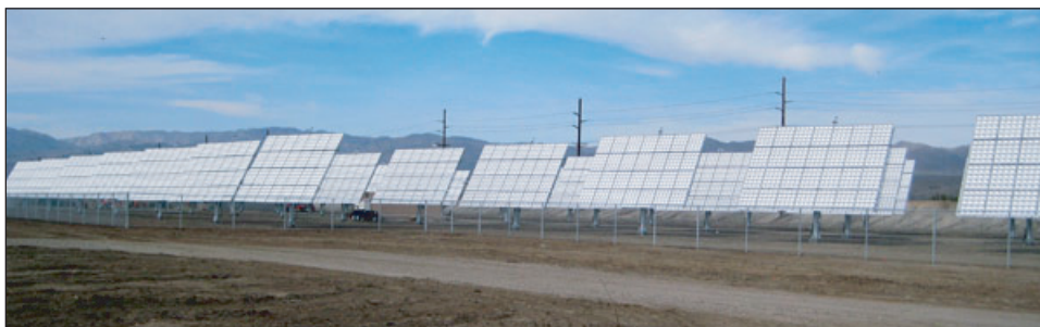
SolFocus' CPV panels at the Coachella Water Reclamation Plant.
